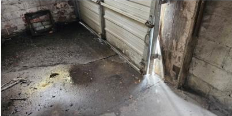
INTERIOR- WATER DAMAGE AND MOLD
