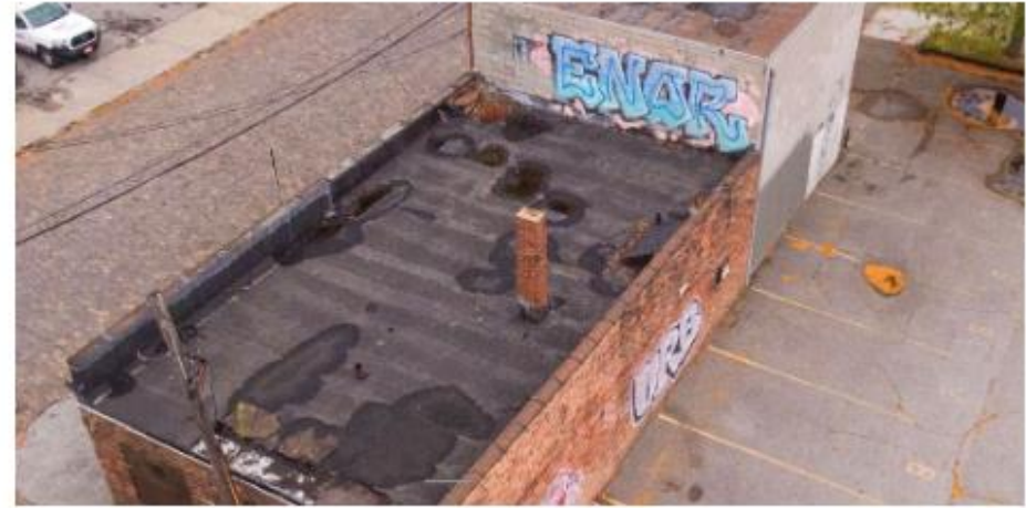
EXTERIOR- ROOF PENETRATIONS AND GRAFITTI
